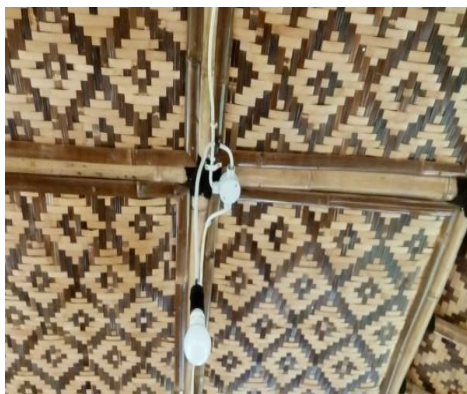
Fig. 9 Unstandard Installation Repair
