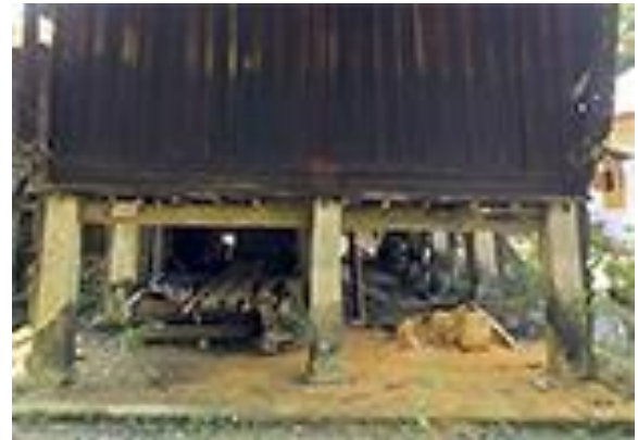
Figure 7. Girders construction of the Bawi Malay Tribe Lontiok house Source: Personal documentation, 2022
